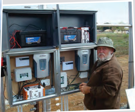
JVA Security Installation, Africa
