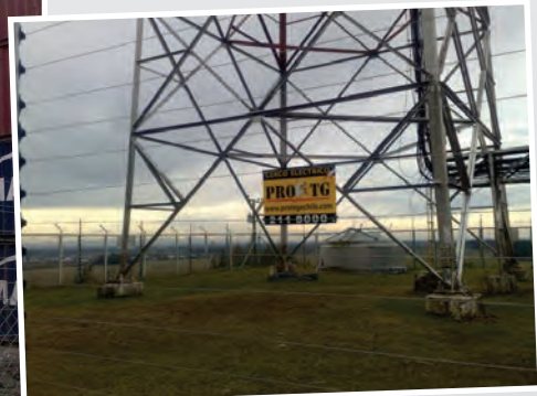
Power Station, Chile
