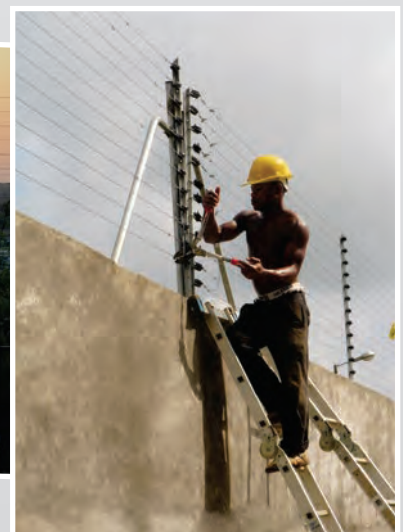
Petro Chemical Plant, Nigeria
