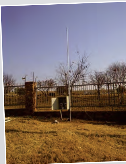
Wireless Repeater Station
