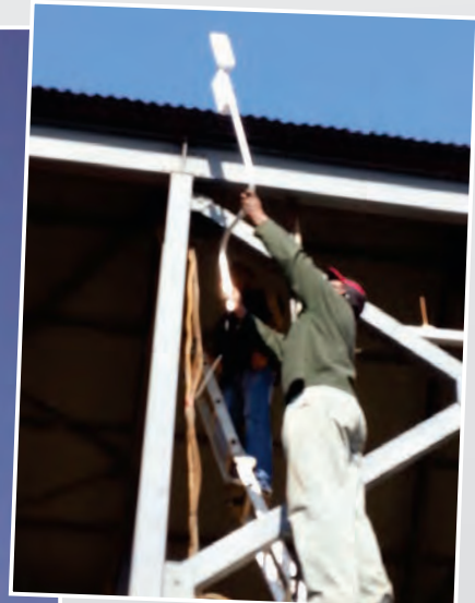
Wireless Repeater at Entrance
