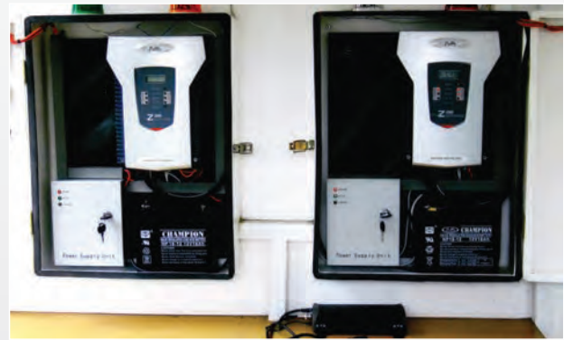
Synchronized System – Internal View
